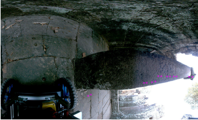
Figure 12. Occluded 3D points. Several 3D points scanned by laser scanner are not observed by omni-directional camera due to occlusion by the pillar
